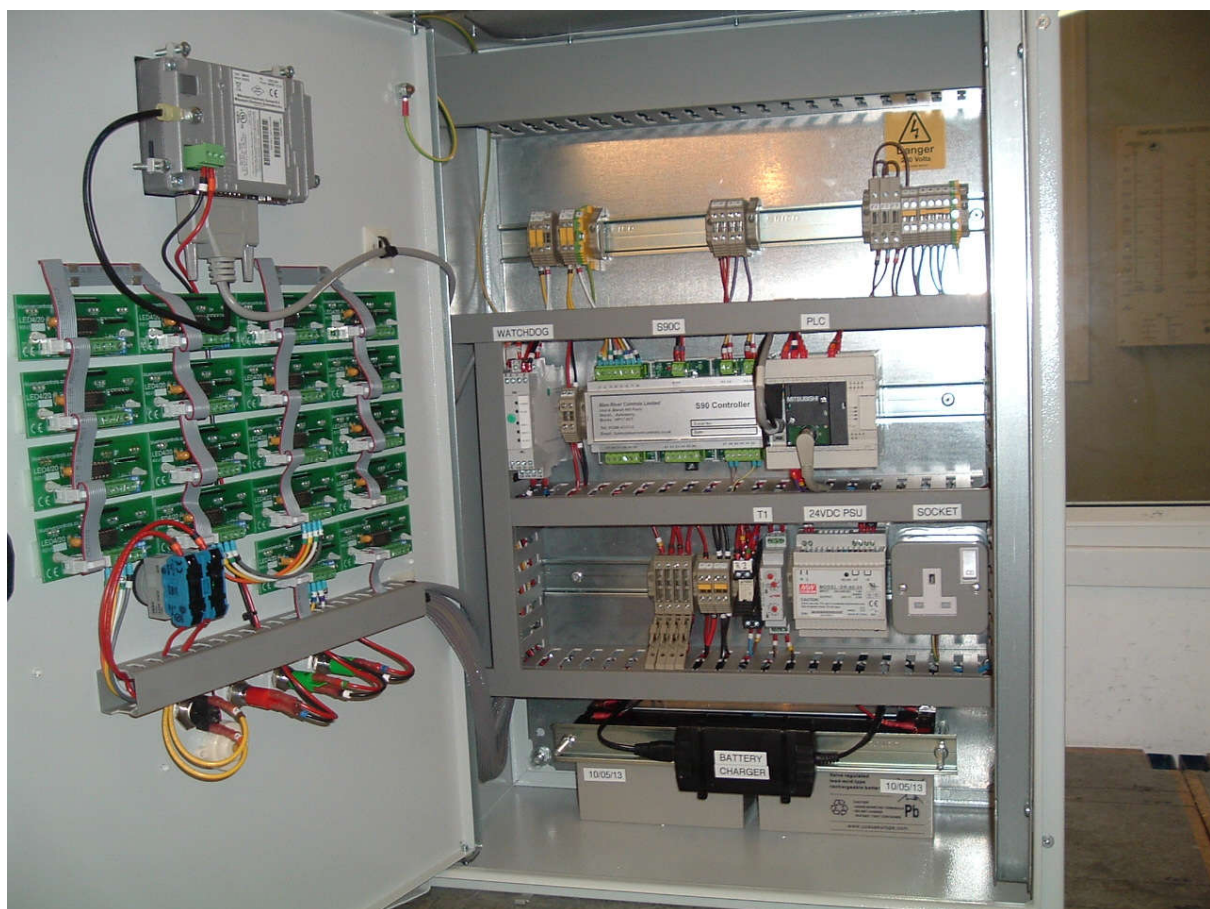
Picture of a typical PLC Addressable Panel
